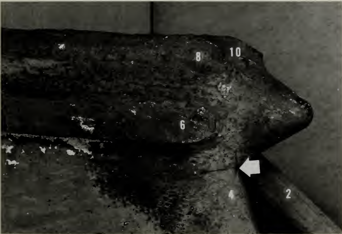
Figure 3. Upstream portion of Howell-Bunger Valve No. 1 showing crack in vane 4. Vane numbers are shown. X 1/2
